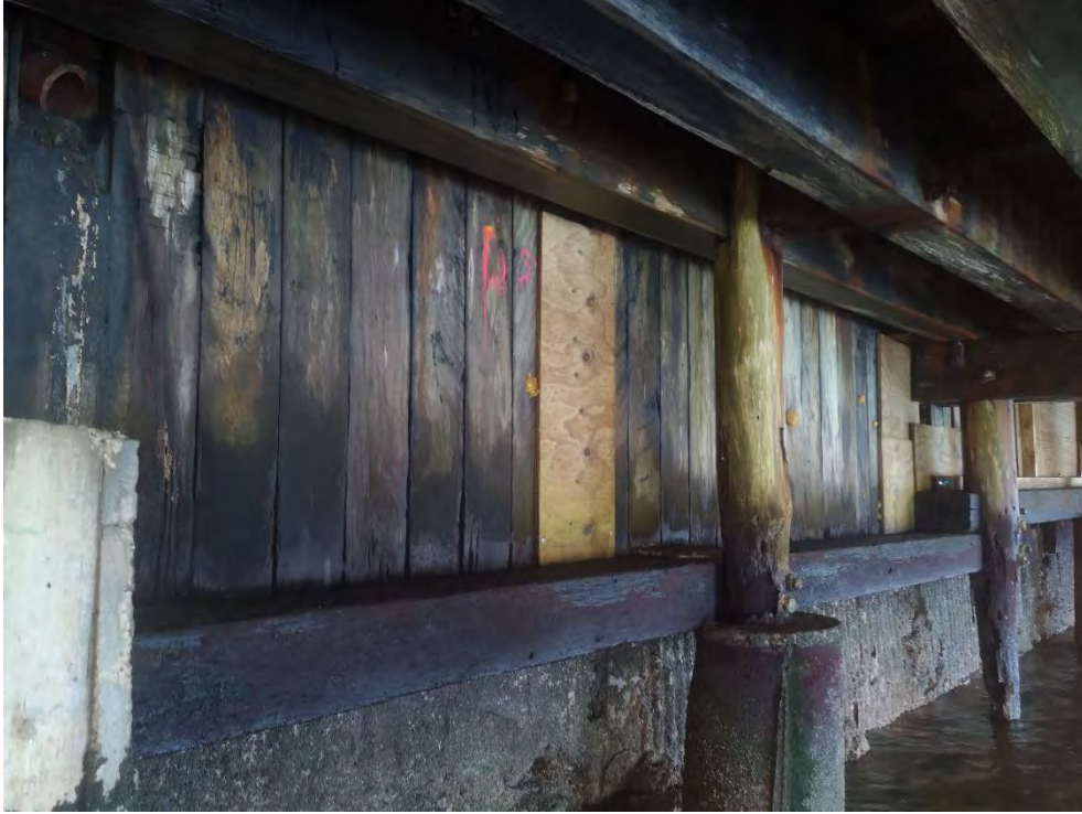
Photograph 15 & 16: Condition of timber railings between access point and Void A. Photos taken above 22/06/2020 and 10/10/2019 below. Damaged pile (void space D – foundation to the North) at location indicated by red circle is pictured in Photograph 16 is no longer observable after securing new plywood facing.
