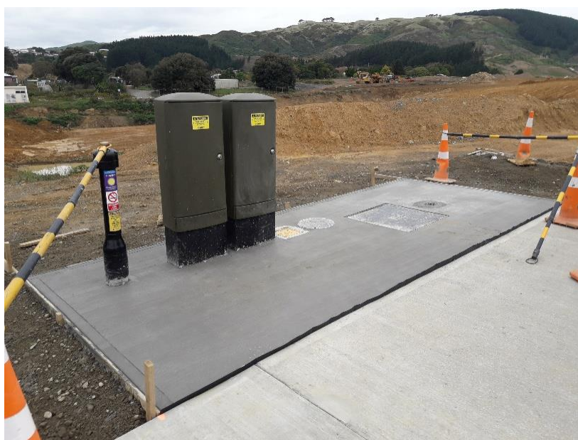
Photo 1: Examples of small above ground equipment
