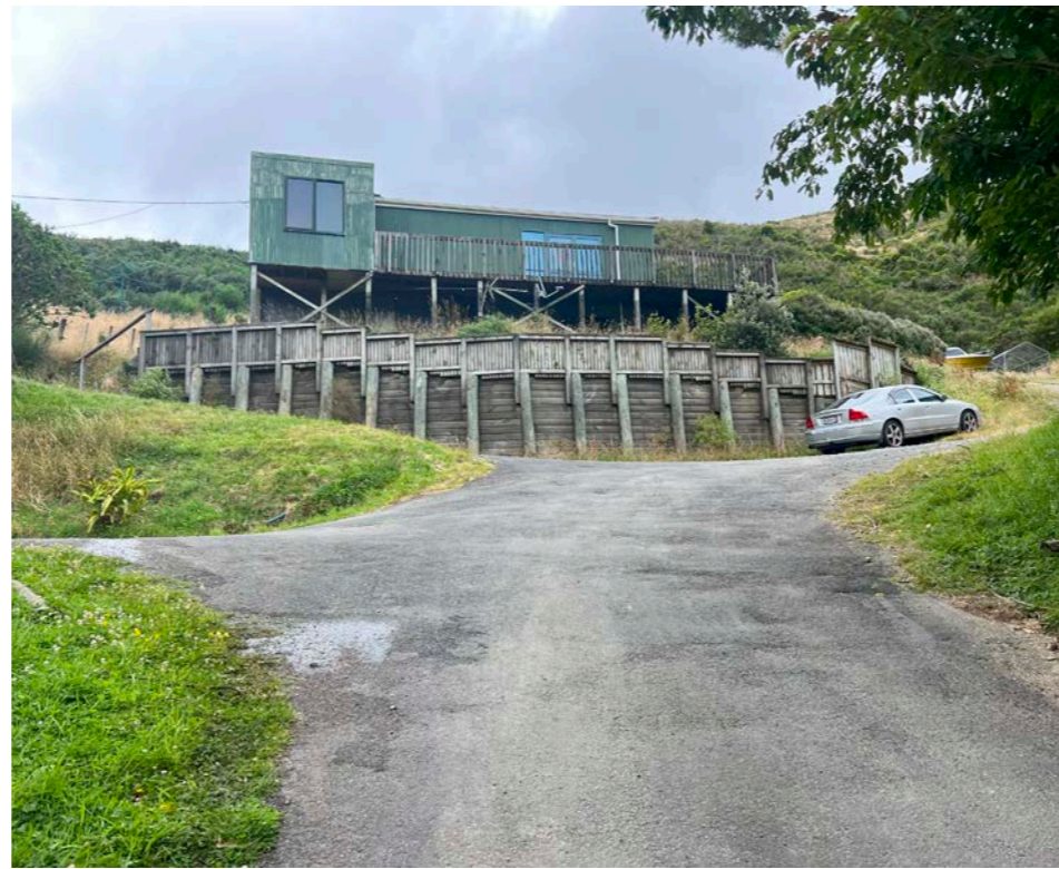
B There are 3 existing dwellings on the site in various states of repair. The site also provides access to two residential properties at 173 and 175 Parkvale Road.
