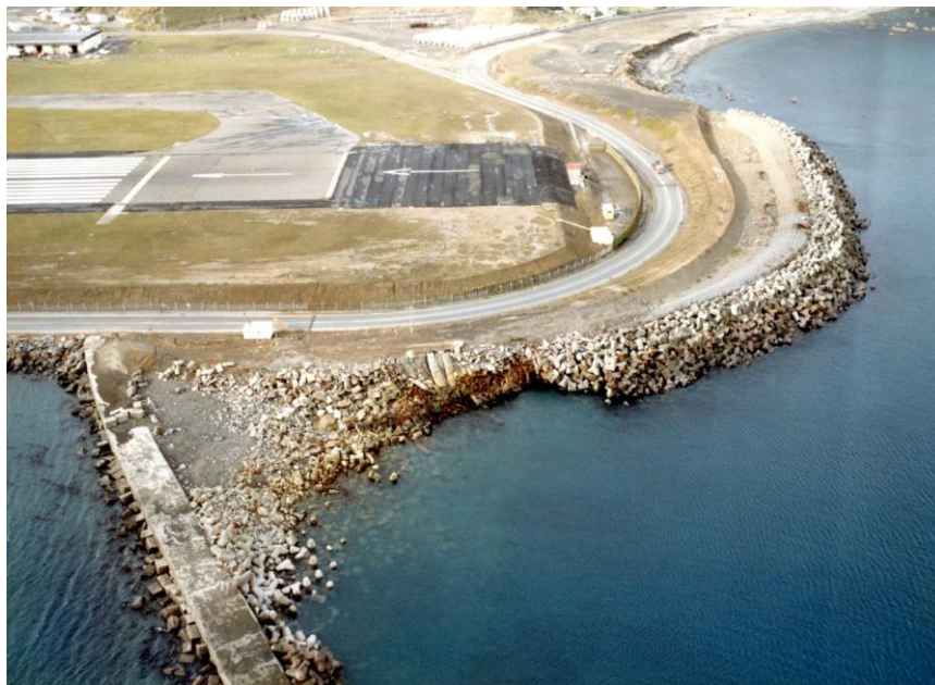
Photo 8: June 1983 seawall breach
