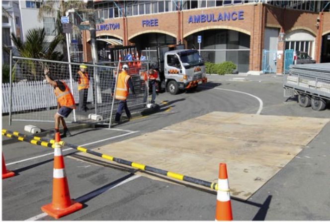
A sink hole in Hobson St
