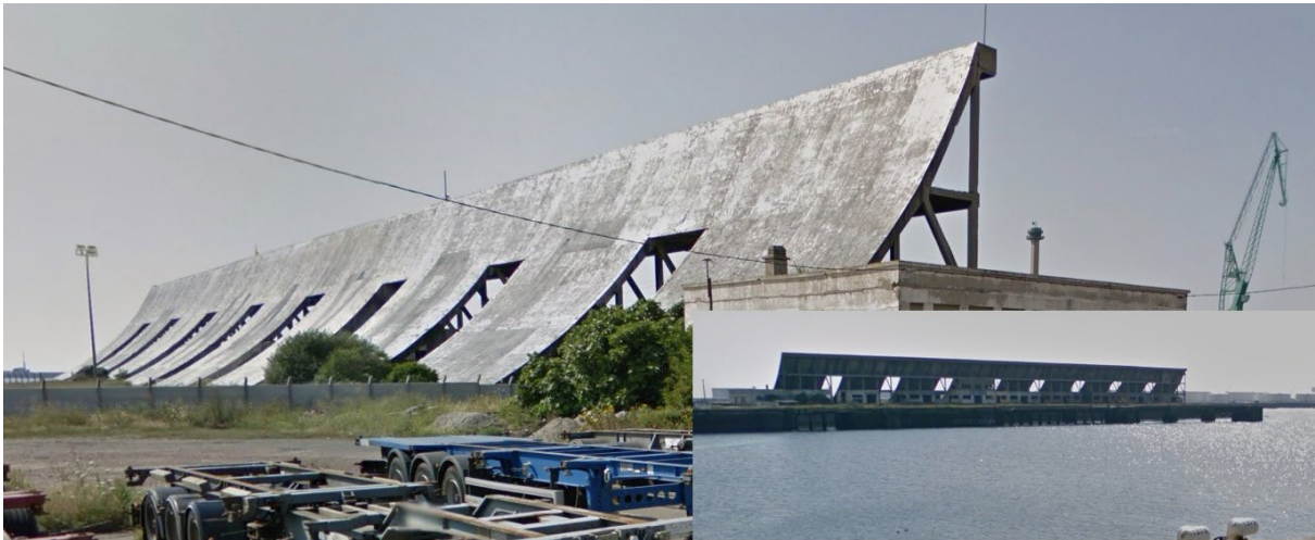
Figure 55 Protection of the boarding quay at Le Havre: concrete springboard ( h = 20\text{ m} , length = 240m) – if this was solid, it is large enough to redirect wind flows
