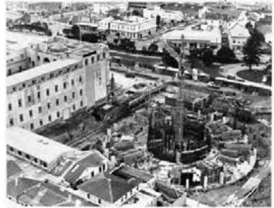
Construction of the Beehive underway in 1971. It would take another decade before it was finally completed. (PAColl-6301-83, ATL)
