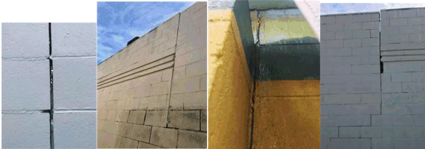
Structural Damage to block southern wall.
