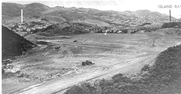
Figure 5: Works in progress, 1949, to transform the Liardet Street tip into a 7 ½ acre playing field - now part of Macalister Park.
