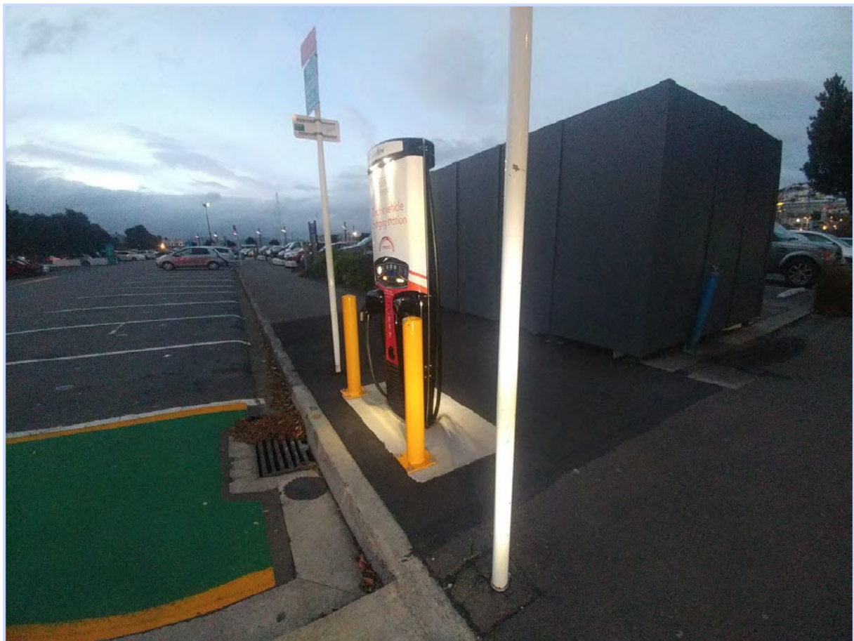
Electric car charging station. Wellington, New Zealand.
