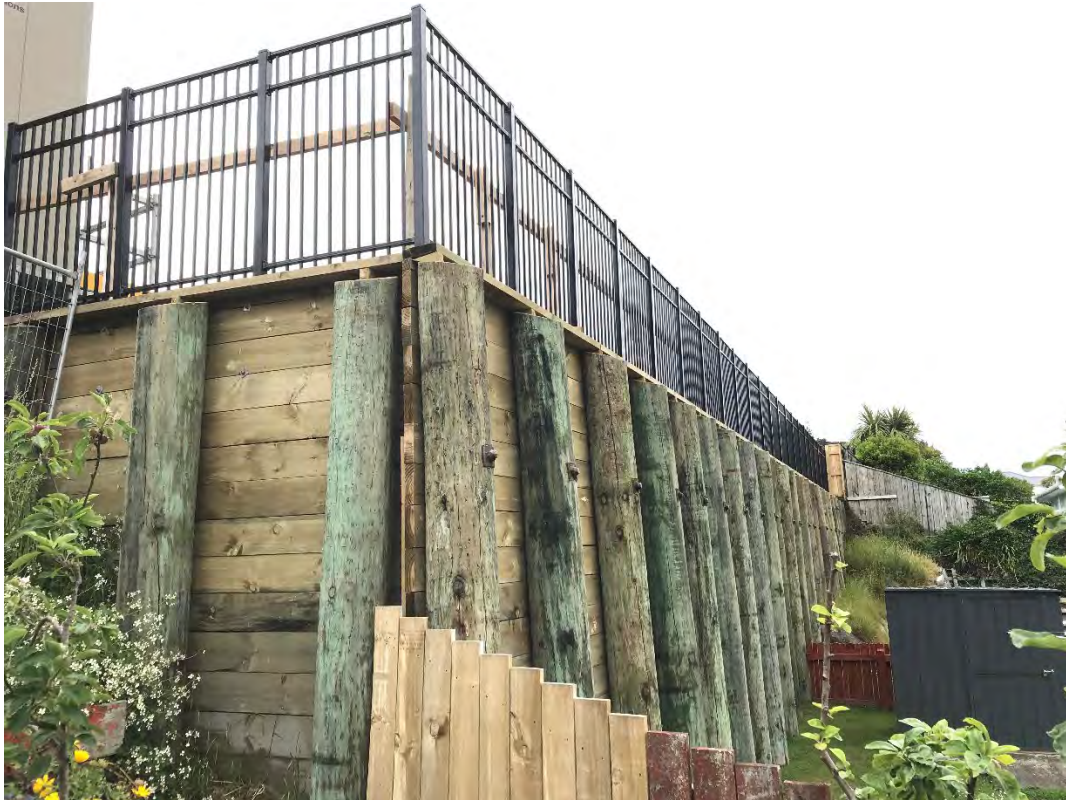
Image 3 – the new retaining wall at the north-west corner of the site. This significant structure allows maximum use of the site for housing.
