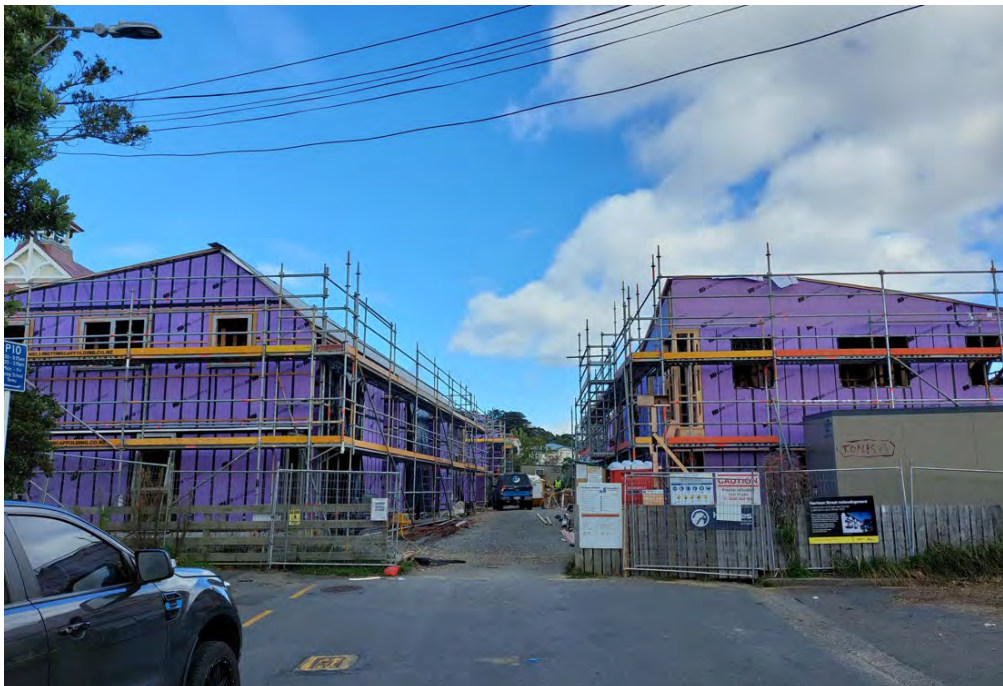
Image 6 – view from the entry to the site, all blocks will be weather tight in the next few weeks.
