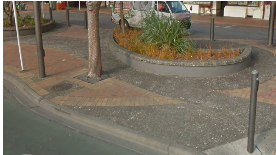
Courtenay Place paving is in a poorer condition than Willis and Lambton Quay, with dated features in exposed aggregate as well as complex header patterns.
