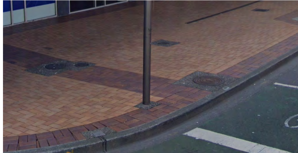
Recently changed areas like near Taranaki Street are in good condition. Kerbs have a narrow form - 150mm wide and are often in poor condition.
