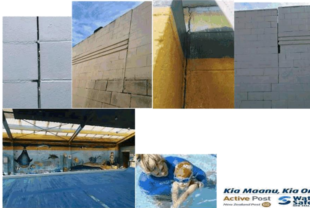
Structural Damage to block southern wall.
