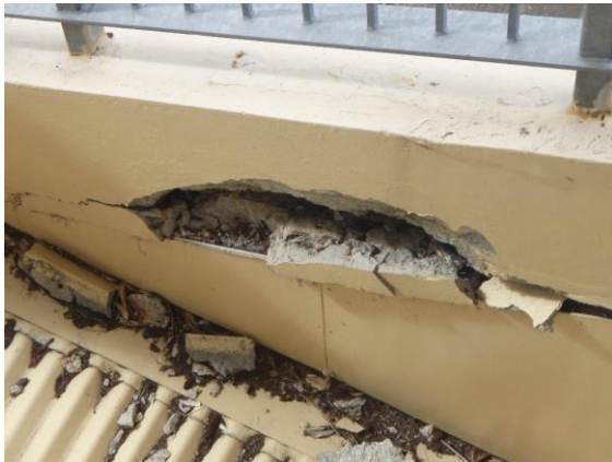
Spalling due to reinforcement corrosion
