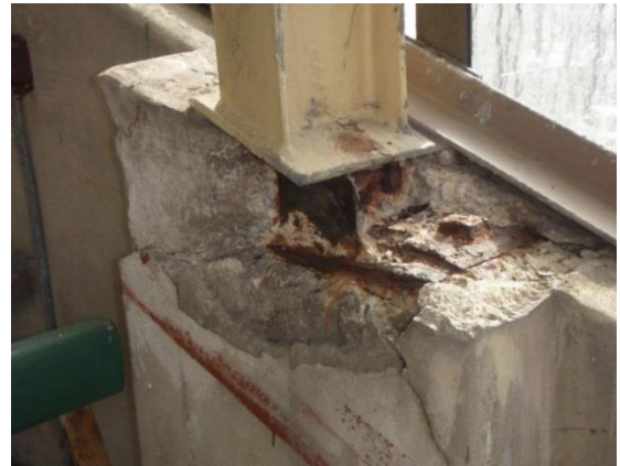
Typical corrosion of roof support column base
