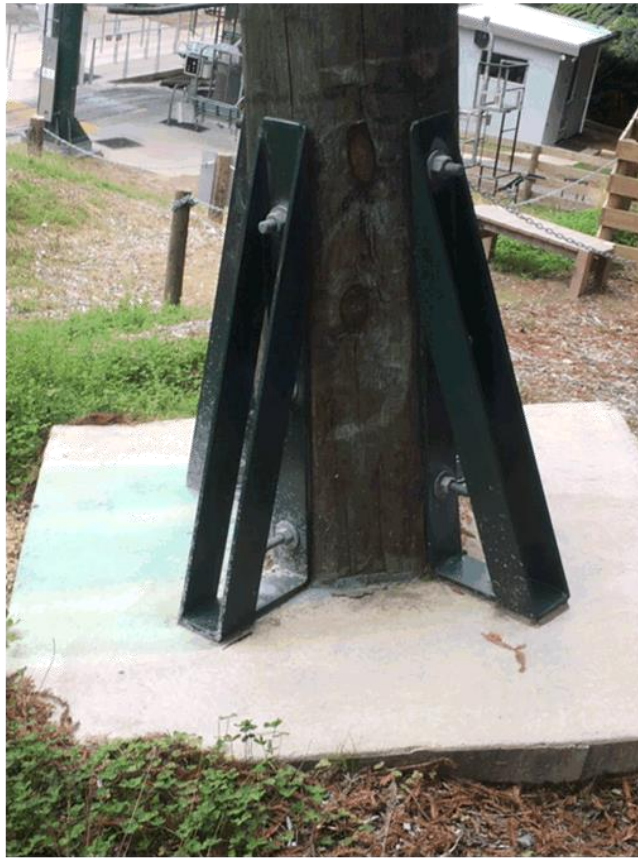
Figure 14: Alternate pole footing option. This requires less excavation and soil removal and simply requires a 500mm thick concrete pad to be laid. Note: This is an option for this project but not until proper design projects have been completed would this type of detail be confirmed.
