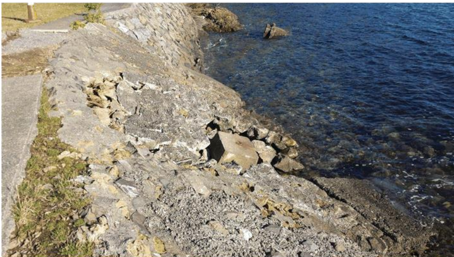
Damaged area of Southern bay
