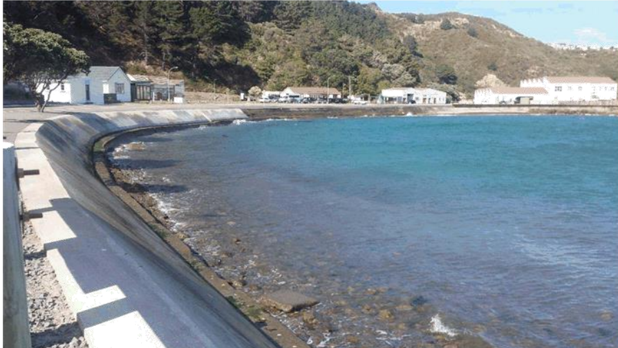
The Northern bay showing recently treated sea wall area (foreground) and untreated sea wall area in distance
