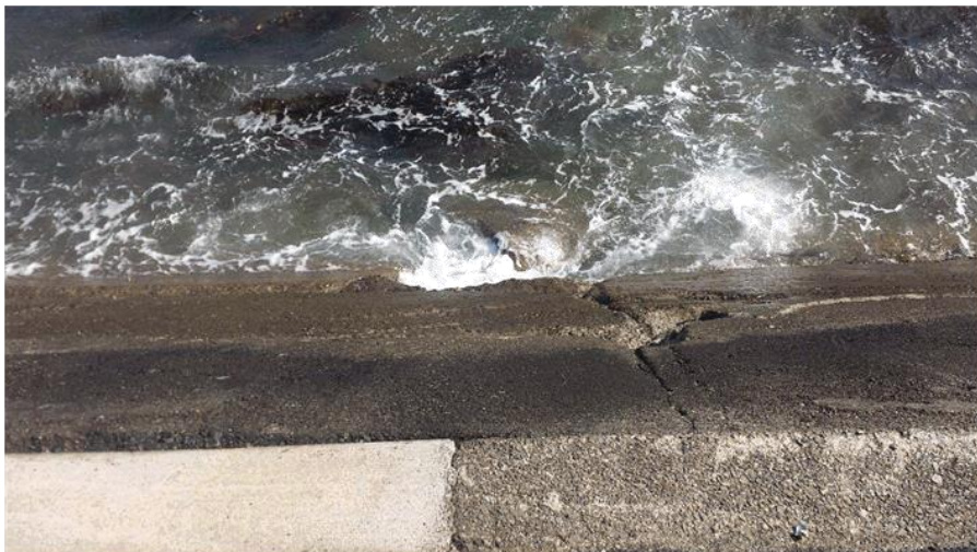
Damaged portion of untreated area of Northern bay sea wall
