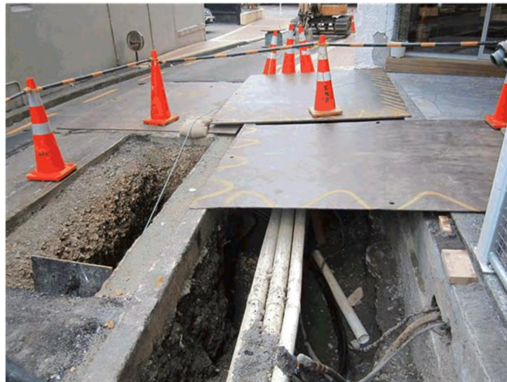
Image showing shallow power services. Photo taken on Lombard Lane
