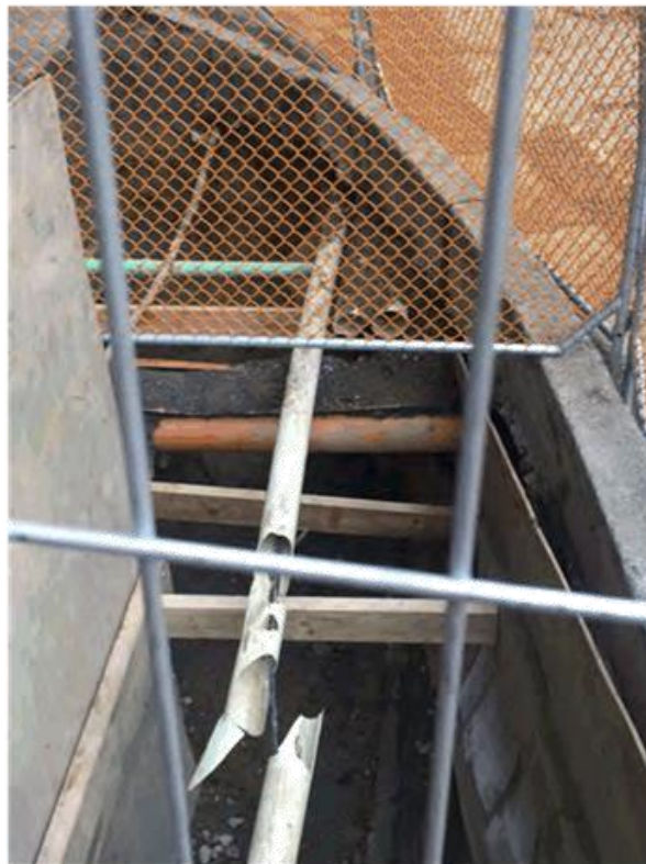
Image showing shallow power services. Photo taken on Lombard Lane
