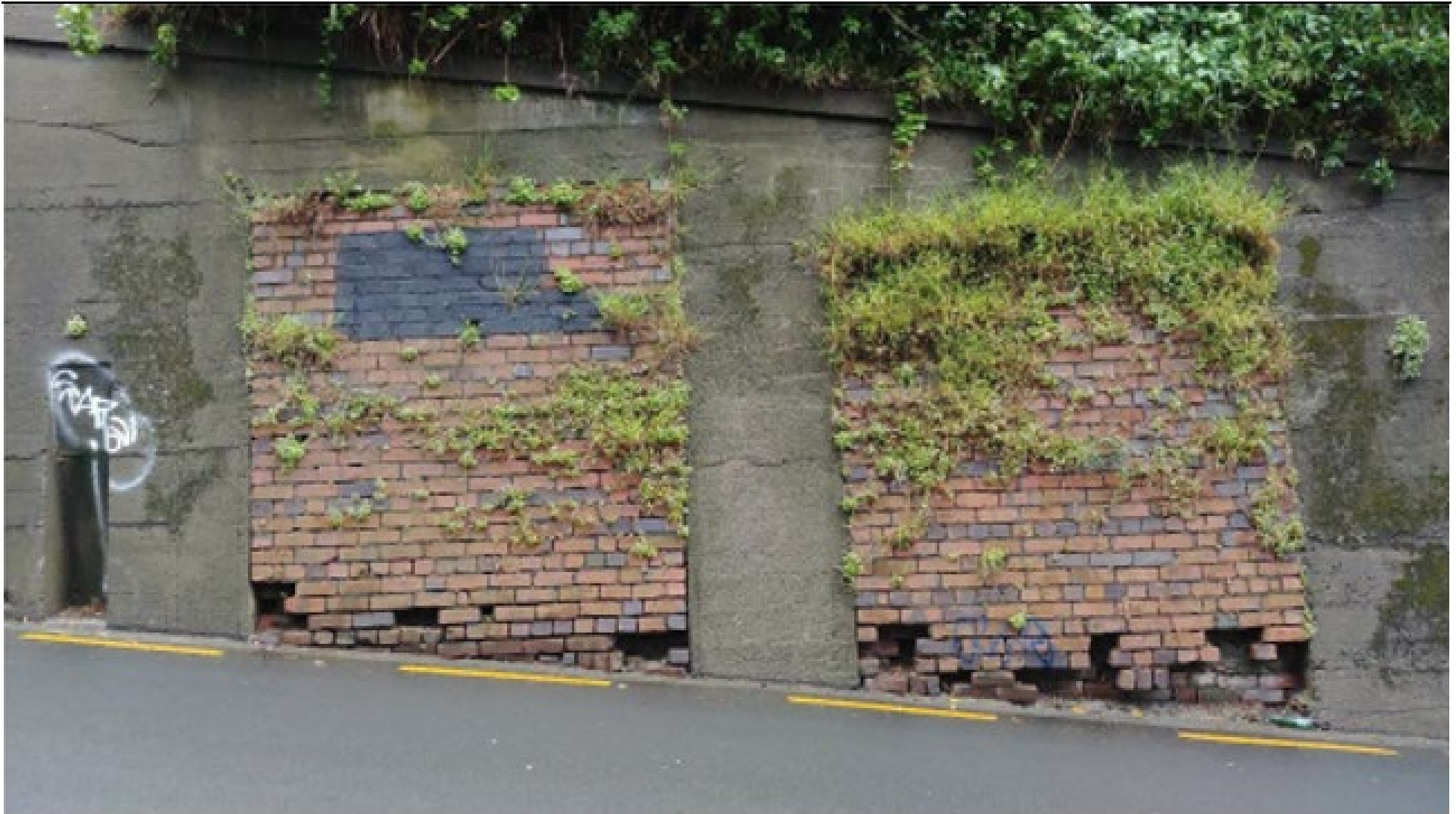
Photograph 12 - Asset 647: Mass gravity, loss mortar
