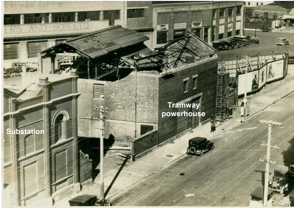
Illustration 22: Demolition of Old Tramway Power House Wakefield street ca 1926 (Wellington City Libraries 50002-3-75)
