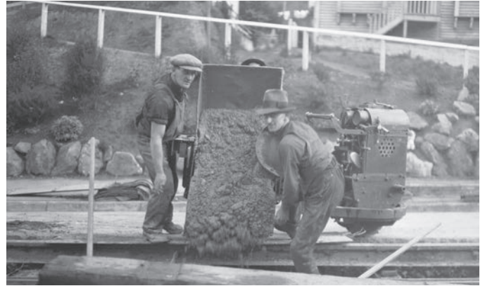
Aro Street, workmen pouring concrete out of tipper on Lister truck, between newly laid tram rails, 1930. WCC Archives 00146-1-30
