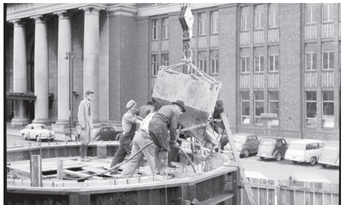
Construction of underground pumping station, railway station, 1954. [columns of station in background, men in foreground directing concrete pourer into wooden formwork]. WCC Archives 00158-1-70
