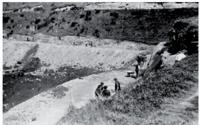
Construction of Alexandra Road, Mount Victoria, in 1930. Workmen are clearing area for new road, using pick, shovel and wheelbarrow. WCC Archives 00157-1-46
